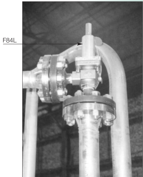
F84L Valve in lube oil service
